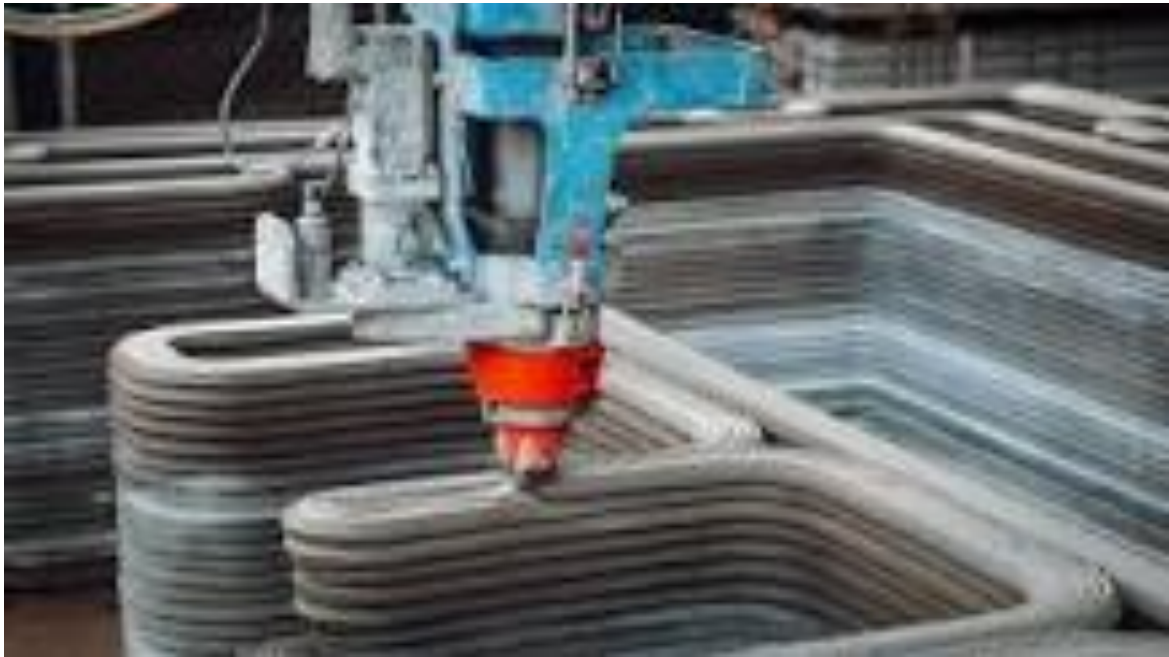
Figure 12: 3D Concrete Printing Process with the Nozzle Extruding Mortar Layer by Layer
