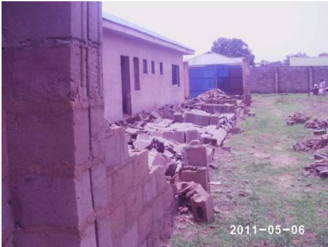
Plate V: Collapse Fencing Wall by Rainstorm
