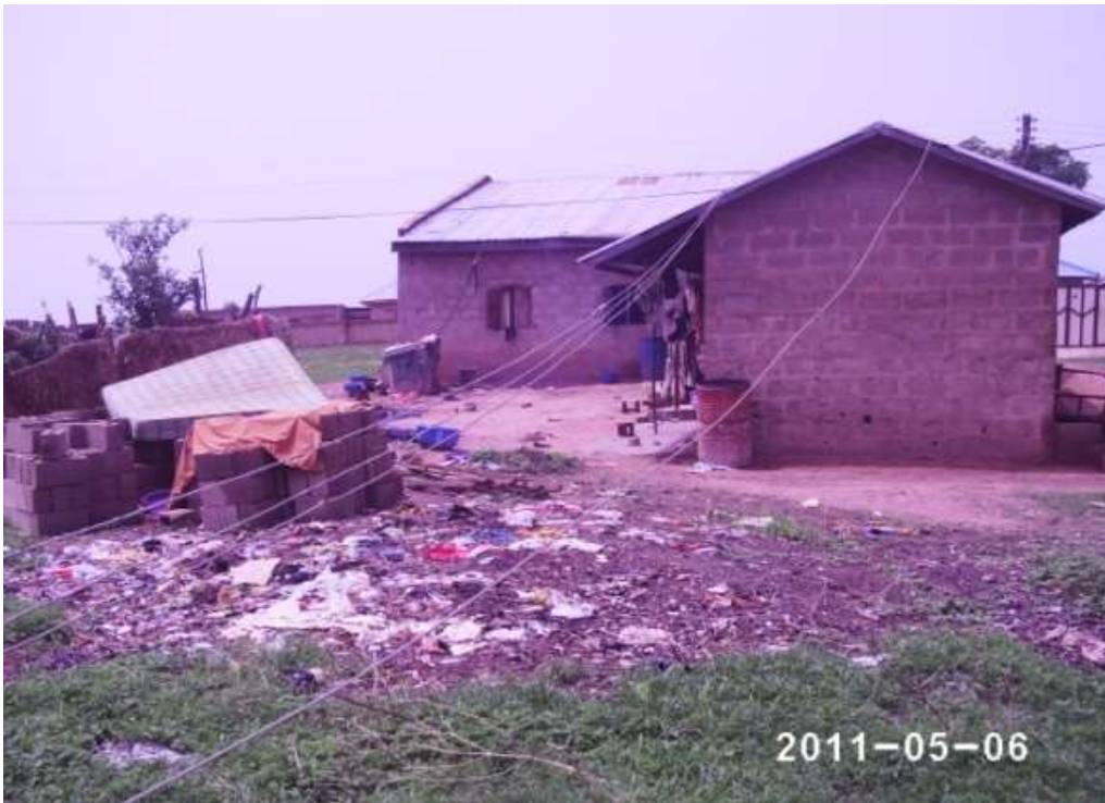
Plate VI: Collapse Electric Cable on the Roof After Rainstorm
