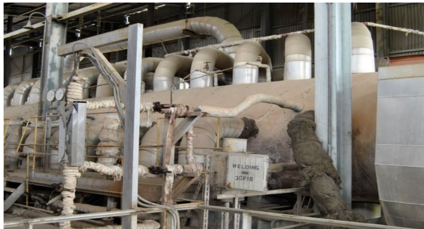
Figure 2: Boiler Drum (Ajaokuta Steel Power Plant)
