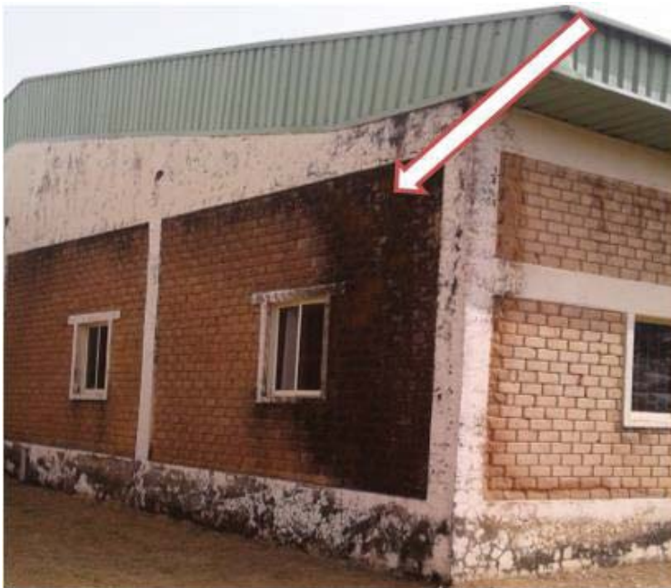
B.1(b): The vertical wall shown with a pointer has dark patches as a result of undrained water from the cladding
