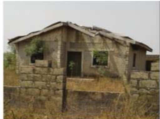
A.1(b): Total failure of load bearing including sinking floor
