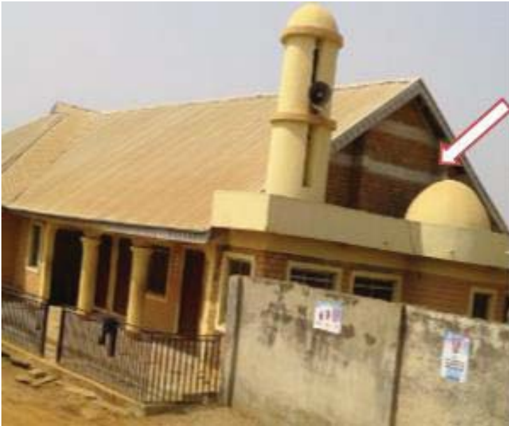
B.1(a): The gable end shown with a pointer collapsed and re-built by introducing vertical pier in the walls
