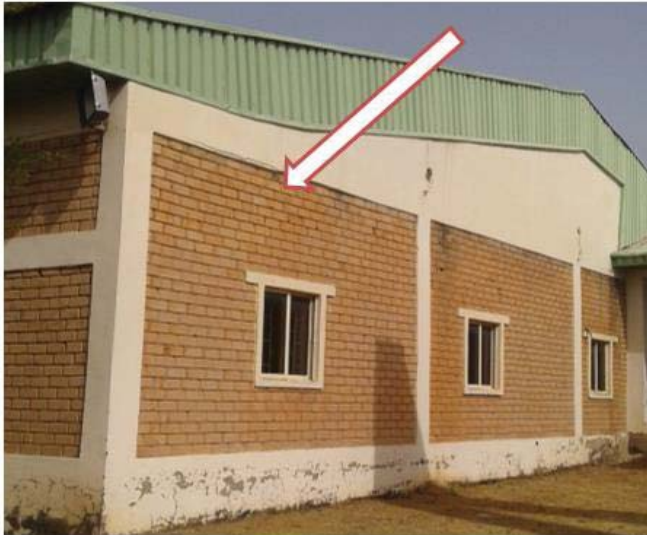
B.1(c): The vertical wall shown with a pointer has caved-in. Could have been prevented if lintel was introduced at window level
