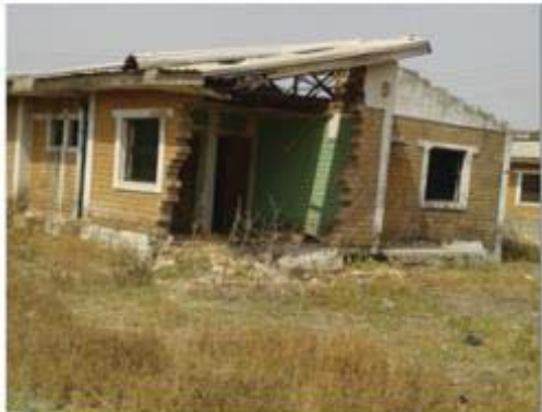
A.1(a): Total failure of load bearing walls and all fabrics of the building
