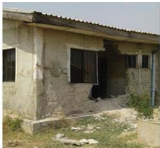
A.1(e): Collapse of external walls and internal partitions
