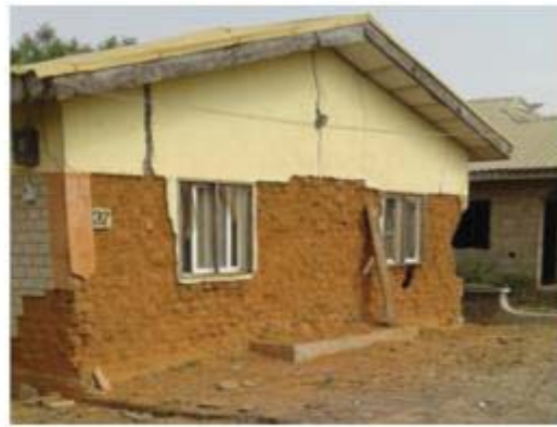
A.1(d): Visible cracks on walls including spalling and eroding wall by rain
