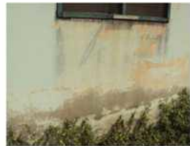
c) water run marks on windows
