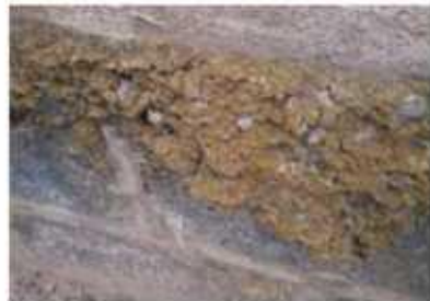
i) mould growth on wall
