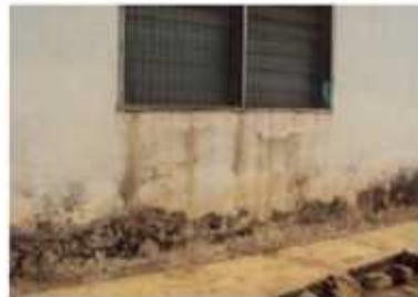
f) Water run marks on window
