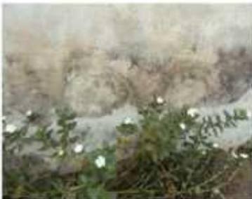
g) Damp at the base of wall
