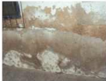
e) Surface efflorescence
