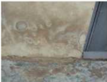
d) Surface efflorescence
