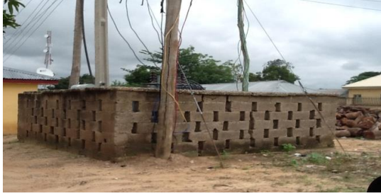
Transformer and road network
