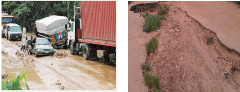
Plate 10: Failed road sections along Minna – Tegina and Tegina - Makera federal road
