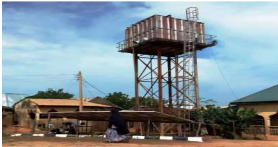
Plate III: Solar-powered water system
