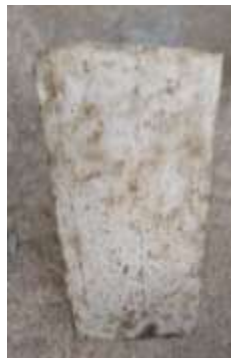
(b) The old concrete prism sample halved at 30° (halved 100 x 100 x 200 mm) As Cast (smooth) surface
