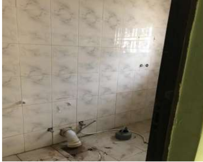
Plate 4.2: An example of a damaged toilet facilities
