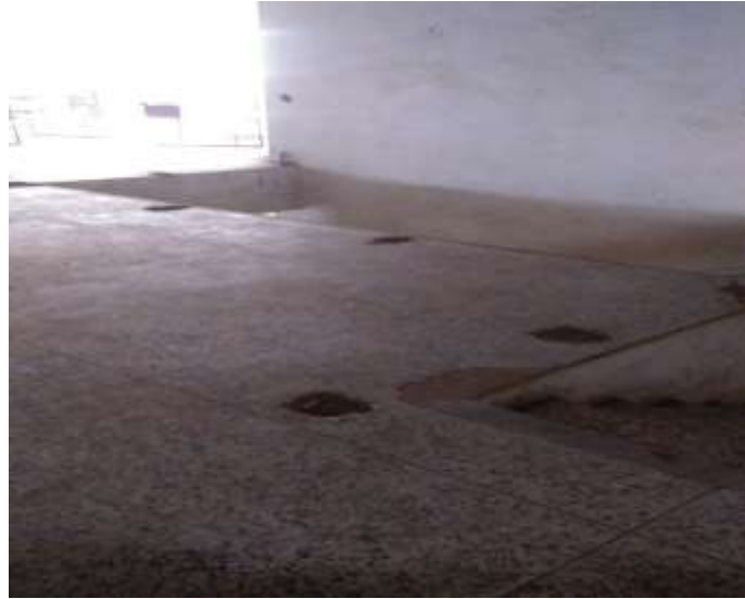
Plate 4.4: An example of a damaged floor
