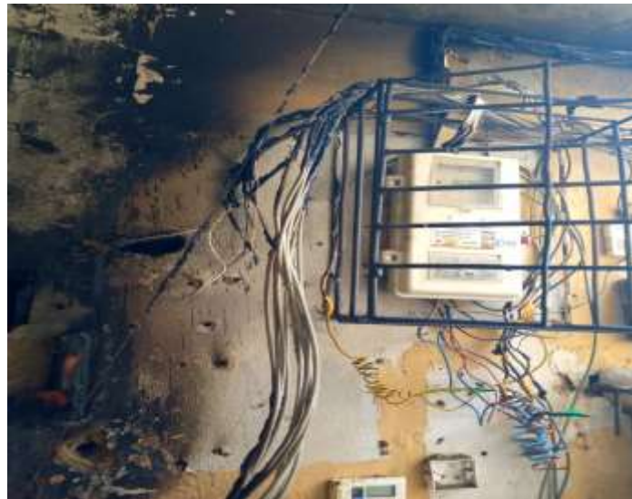
Plate 4.3: An example of a damaged electrical facilities
