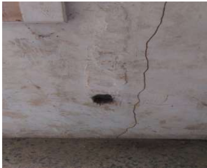
Plate 4.1: An example of a structural crack in a wall
