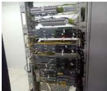
Plate VI A Rack of Microwave Radio Indoor Units for NEs.
