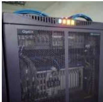
Plate IV OptiX900 (Fibre Termination Equipment, Vendor: Huawei)
