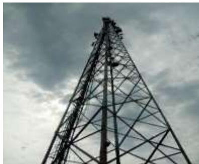
Plate V Tower (For Mounting RF, Microwave Antennas and Terminating Cables)
