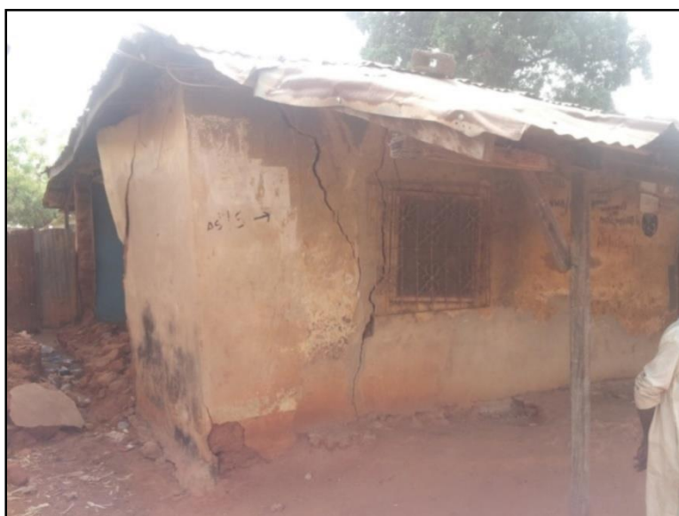
Plate I: Building With Collapsed Wall in the Study Area
