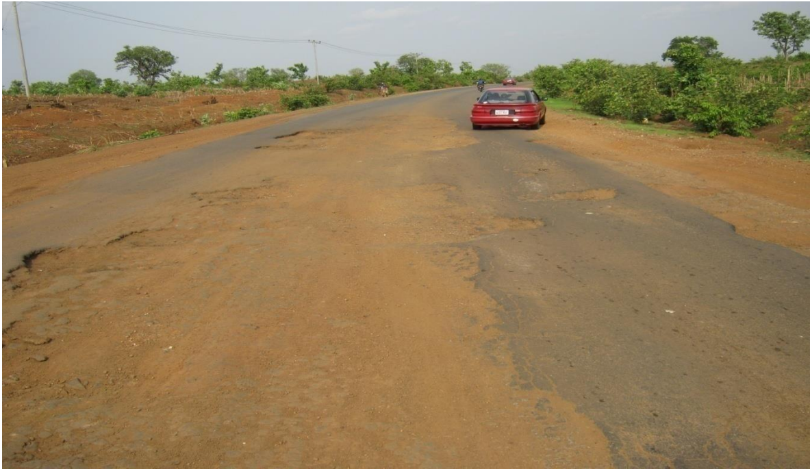
Plate 1: Failed section of the roadway at Mai Wayo Village (Sabon Eregi) along the Minna-Bida road.
