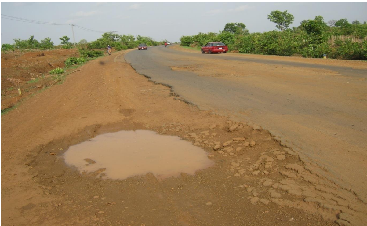
Plate 2: Water retained on the failed section of the road shoulder at Mai Wayo Village (Sabon Eregi) along the Minna-Bida road.
