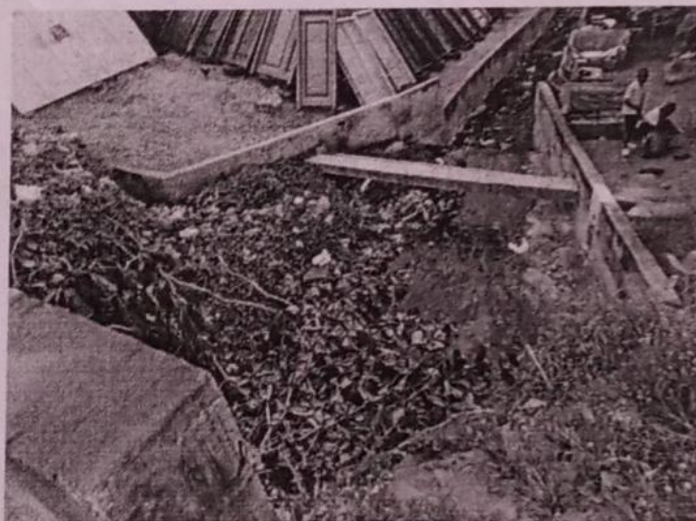
Fig 9: Blocked drainage in Ganaja. Source: Authors
