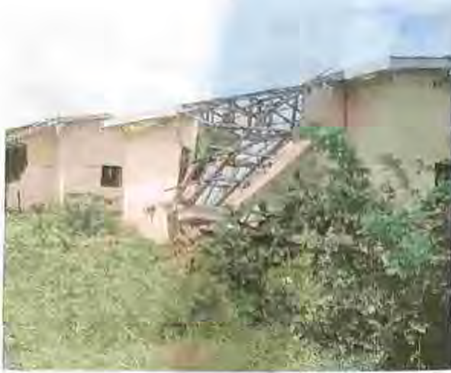
Plate 3 showing a complete collapse of a section of the 2 bedroom: source authors field survey 2010
