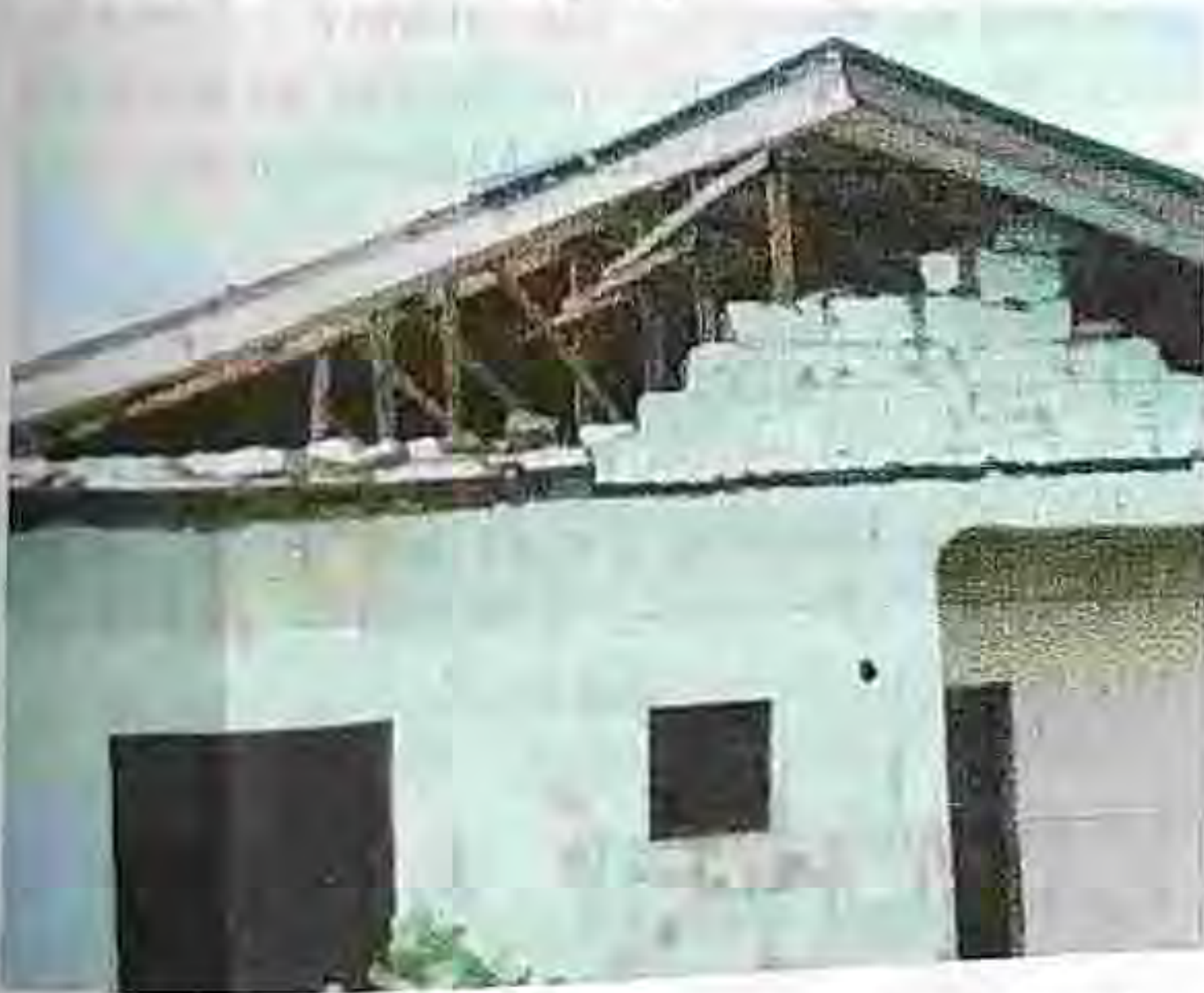
Plate 1; showing structural failures on the walls of 2 bedrooms. Source authors' field survey 2010
