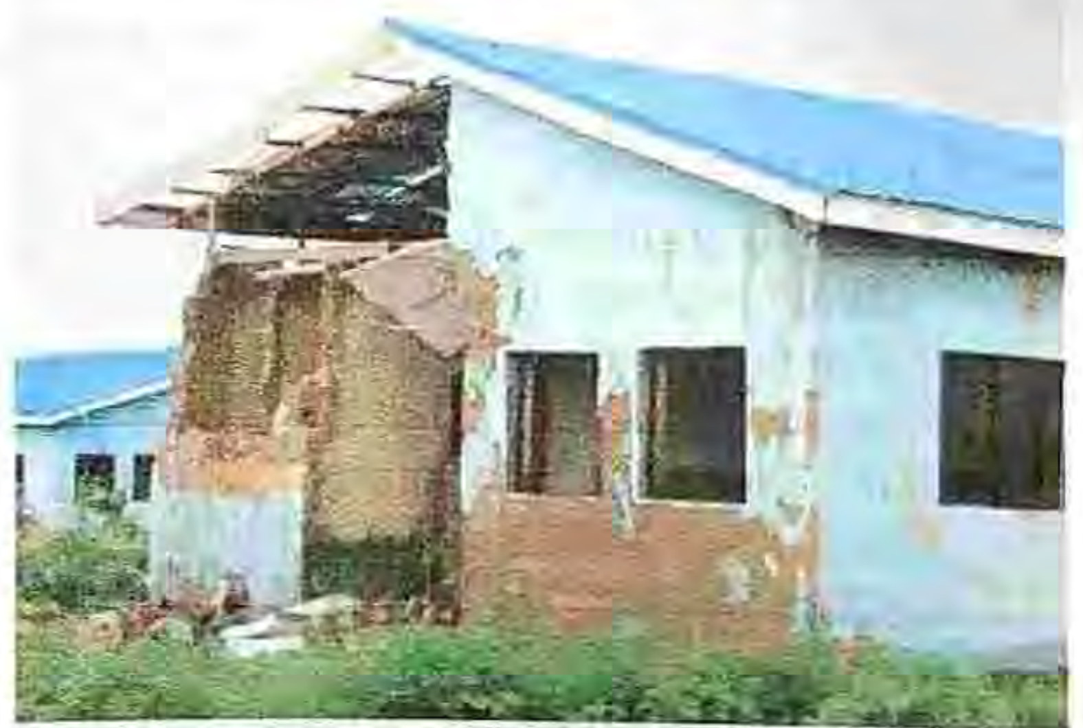
Plate 2 showing a structural failure of wall in 2 bedroom : Source authors' field survey 2010
