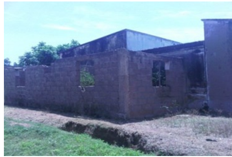
Figure 8: View of the unit
