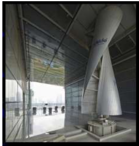
Plate III: A turbine in one of the four intakes in the Pearl River Tower
