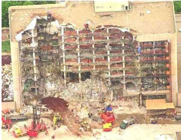
Fig 2.7: Alfred P Murrah Building, Oklahoma City, Oklahoma, April 19, 1995: Progressive damage that is caused directly by the bomb. Source: Building and Construction Authority, 2005)
