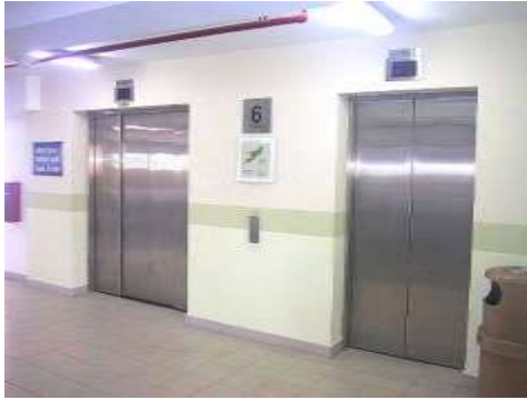
Fig 2.16: Do away with the use of common lift systems (Source: Building and Construction Authority, 2005)
