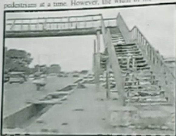
Plate V: Steepness of the Old Pedestrian Bridge in Minna
