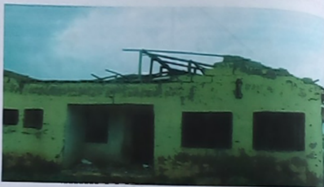
Plate 1: Poorly constructed unit
