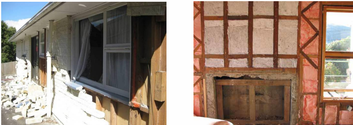
Figure 1. Broken wall claddings and interior linings make an opportunity for installing wall insulation
