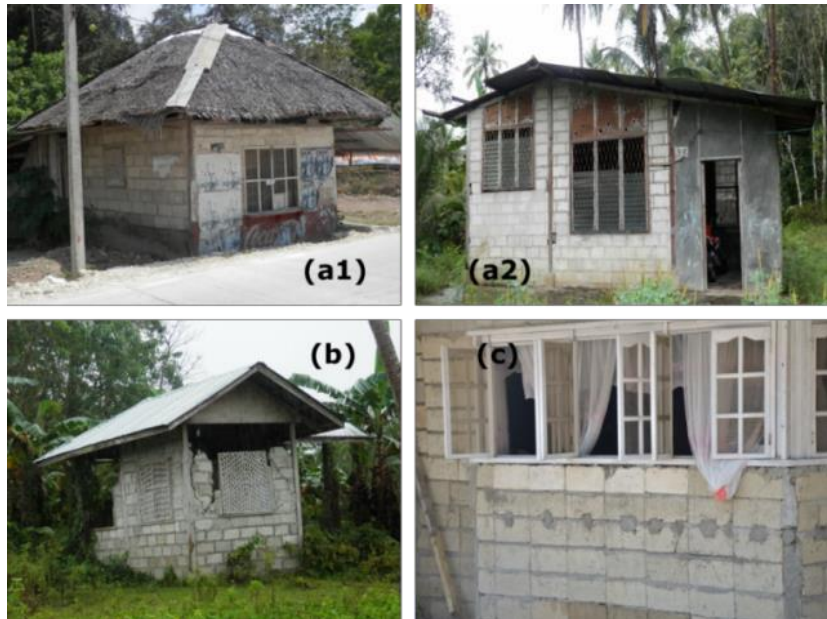
Figure 4. (a) Residential dwellings under the CHB building class; (b) Weak walls due to absence of steel bars; and (c) CHBs piled on top of the other various eras of construction. Moreover, data binning divides the total sample in each building class with respect to intensity contours, construction era and damage states. An intensity value is assigned to every village, depending on its geographical location. The fraction of the total number of buildings for a certain damage state in each intensity level and era are computed.
