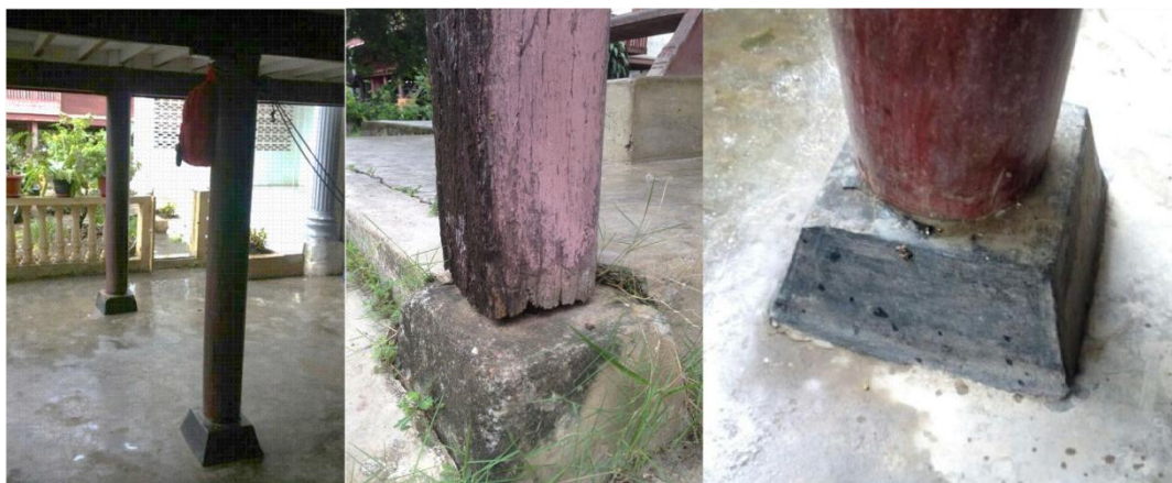
Figure 05. 'lack of foundations - posts resting on concrete plinths'
