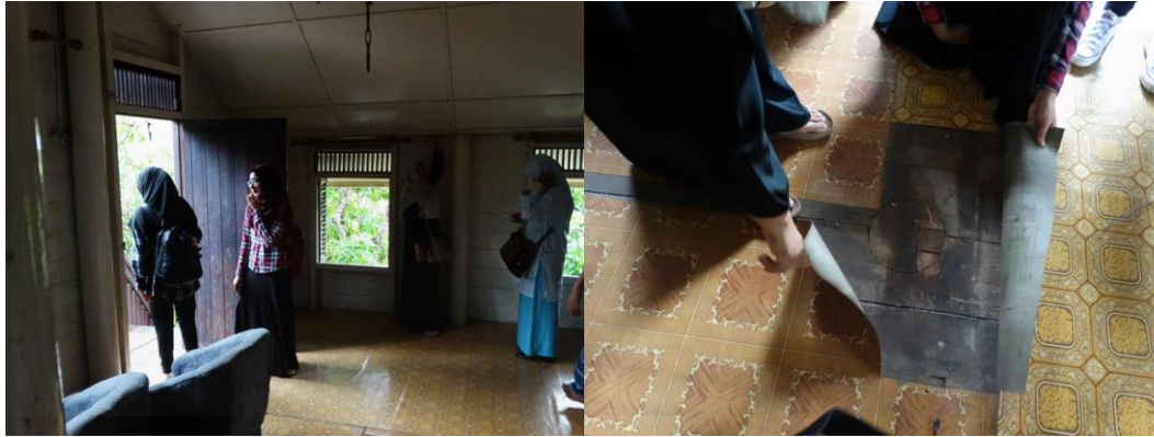
Figure 02. 'structural column from below removed to great more space in the interior'
