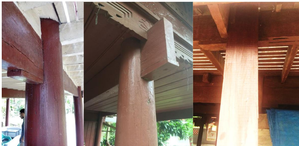
Figure 04. 'Construction joints with wooden wedges that loosen during an earthquake to increase elasticity'
