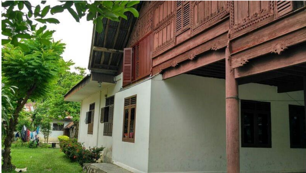
Figure 01. 'Modern addition to existing Rumah Aceh. Enclosing rear bay and extension to rear, clay brick construction with concrete render'
