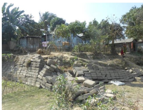
Figure 6 Failing concrete block wall along the north-east corner of the Concernpara settlement – community members have previously rearranged the blocks, such that the current arrangement may not match initial installation. (Author’s own image, 2015)
