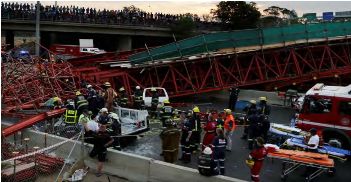
Figure 1: Collapse of a bridge under construction in Johannesburg (Source: News24: online)
