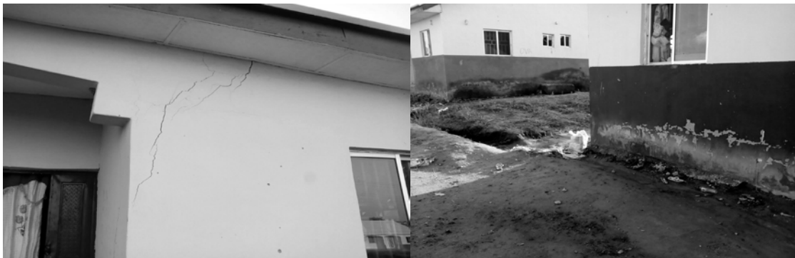
Figure 1(a) and (b) Figures showing visible defects on newly constructed houses for Post-2012 flood victims in Lokoja, Kogi State, Nigeria.
