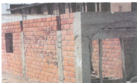
Plate 3: Showing : Building marked for demolition due to encroachment into Road Researvation at Tunga Site Minna.(Source: D.C. Minna 2011)
