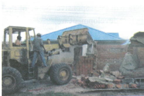
Plate 2: Showing : Building under demolition due to encroachment into Govt's Layout (Illegal Title) at Site MTP 17 Bosso, Old Abattoir Road Minna.(Source: D.C. Minna 2011)
