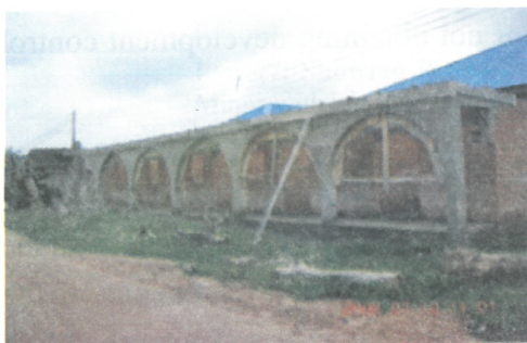
Plate 1: Showing : Building marked for demolition due to encroachment into Govt's Layout ( Illegal Title) at Site MTP 17 Bosso, Old Abattoir Road Minna. (Source: D.C. Minna 2011)
