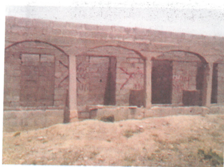
Plate 6: Showing Building under construction along Minna -Bida Road marked by the Development Control for contravening the law. (Source Researcher's field work 2011)
