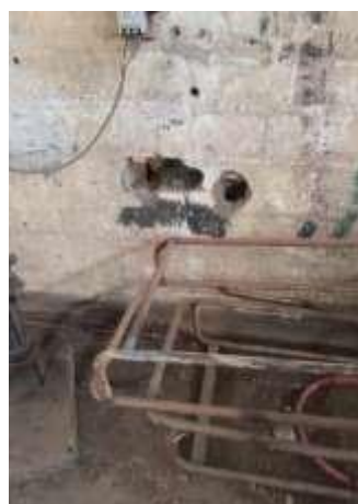
Picture 3: Faded paint and holes on wall
