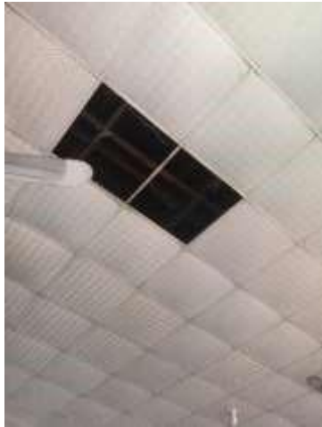
Picture 4: Damaged ceiling
