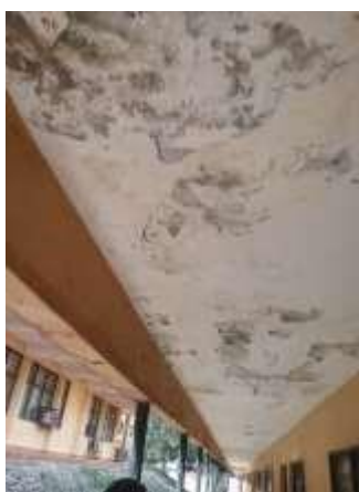
Picture 2: Faded paint and holes
