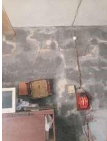
Picture 5: Exposed wire and faded paint
