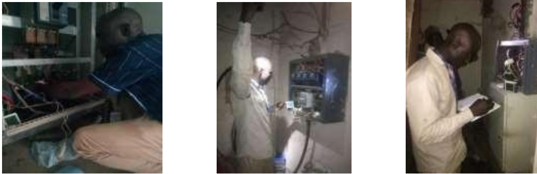
Figure 3.2: Clipping the jack-plug on the live wires at Zungeru Polytechnic and Niger State College of Education administrative blocks the main panel distribution board (MPDB).
