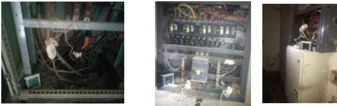
Figure 3.3: Connection at the Zungeru Polytechnic and Niger State College of Education administrative buildings MPDB.
