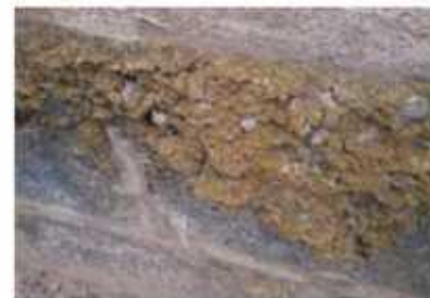
i) mould growth on wall
