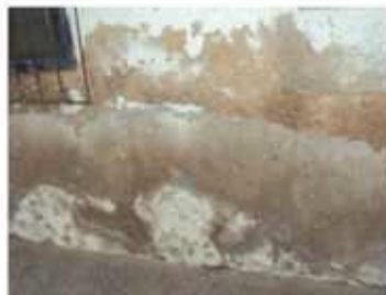
e) Surface efflorescence
