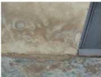
d) Surface efflorescence
