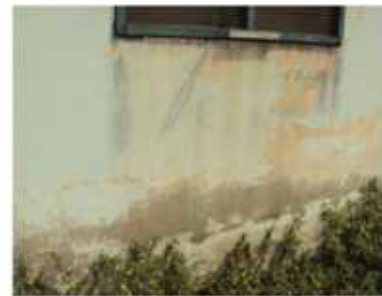
c) water run marks on windows
