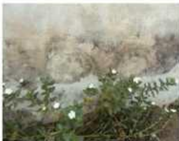
g) Damp at the base of wall
