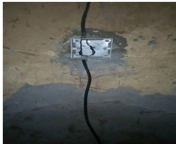
Figure 5: Exposed wires and sockets
