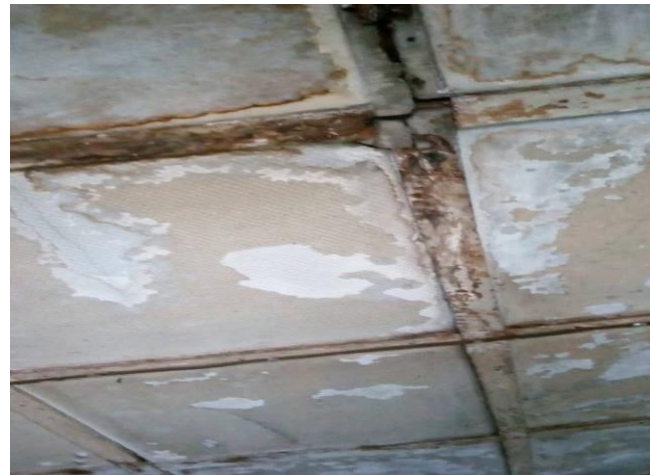
Figure 2: Decay in the ceiling (internal)
