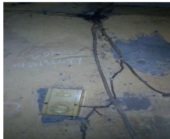
Figure 6: Exposed wires and sockets
