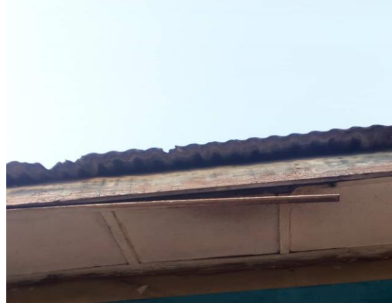
Figure 4: Deterioration of the external ceiling
