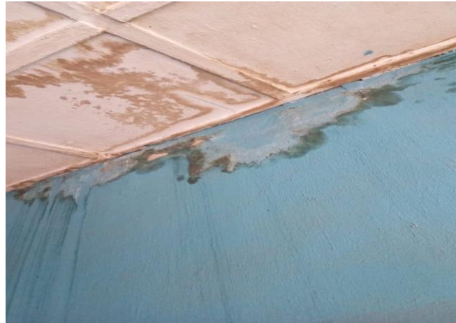
Figure 1: Decay in the ceiling and damages to the paint (internal)
