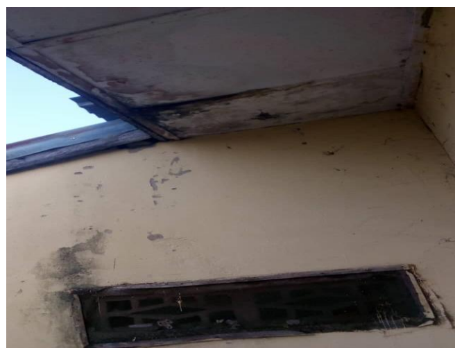
Figure 3: Decay in the ceiling (external)
