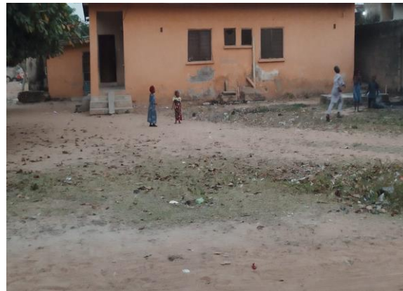
Figure 8: Deterioration of paint and plaster of external walls
