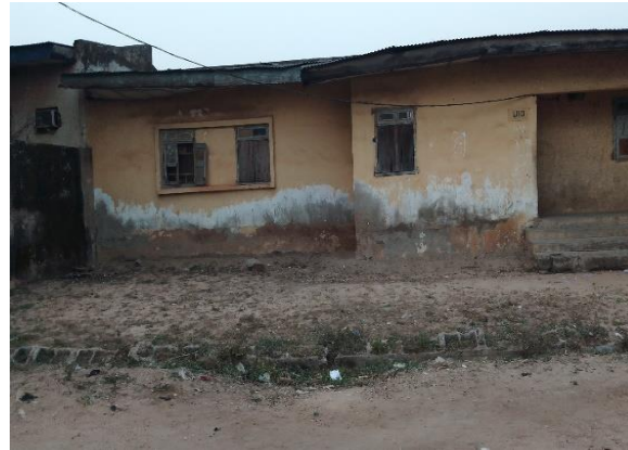
Figure 7: Deterioration of paint and plaster of external walls
