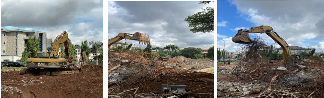
Figure 1, 2 and 3: Pictures showing two operators with the backhoe excavators demolishing and clearing
